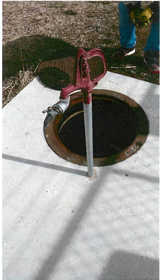
Access to pit where flow meters are for well #1 and #2.
