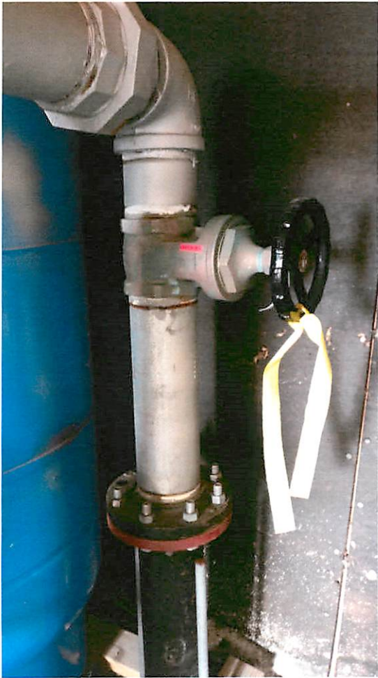
Gate valve well #1
