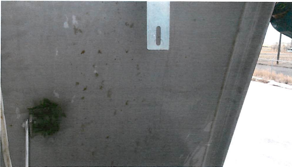
Manhole lid without seal
