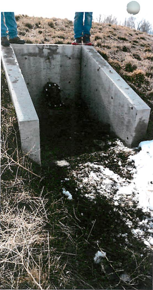
Overflow of storage tank
