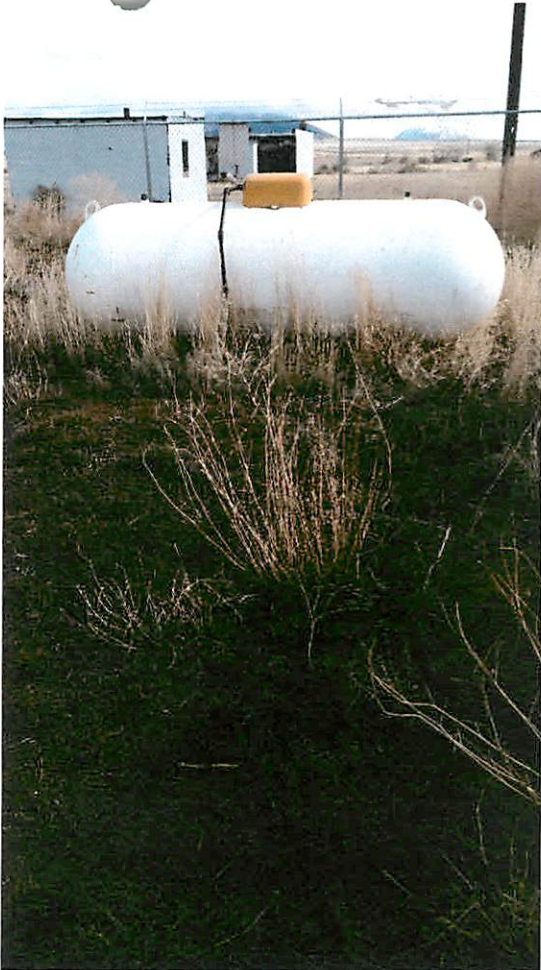
Propane tank for generator
