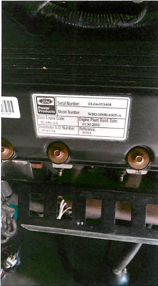
Auxiliary power generator
